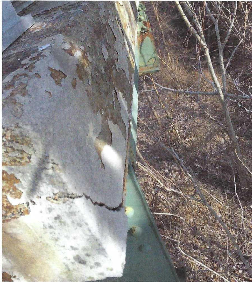
Figure 2 - Southwest end looking downward and east - Spall continuing to end of deck
