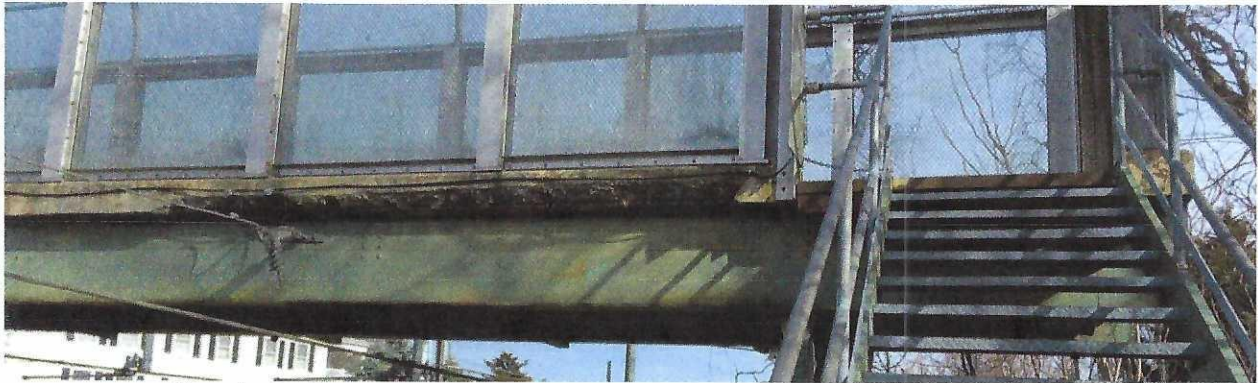
Figure 1 – Southwest end, looking southeast - Spalling of concrete curb element at longitudinal rebar
