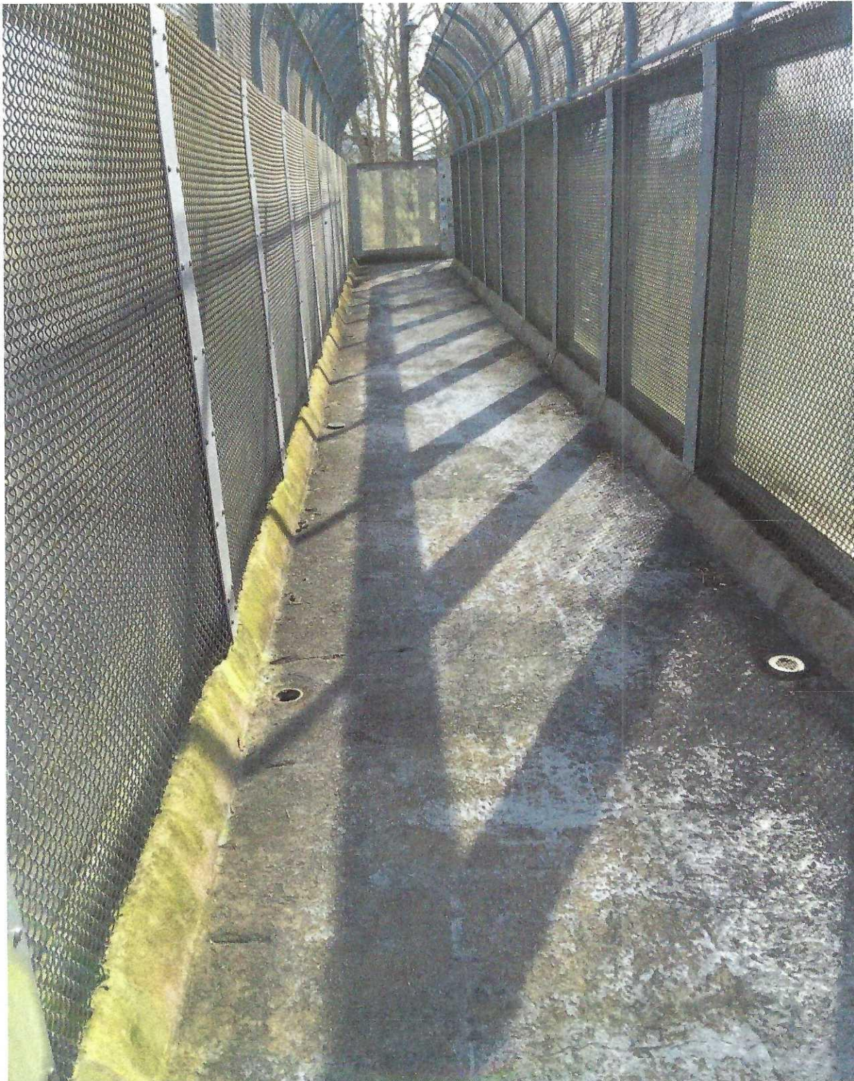
Figure 4 - Deck surface, looking southwest from north end - Spalled/weathered surface
