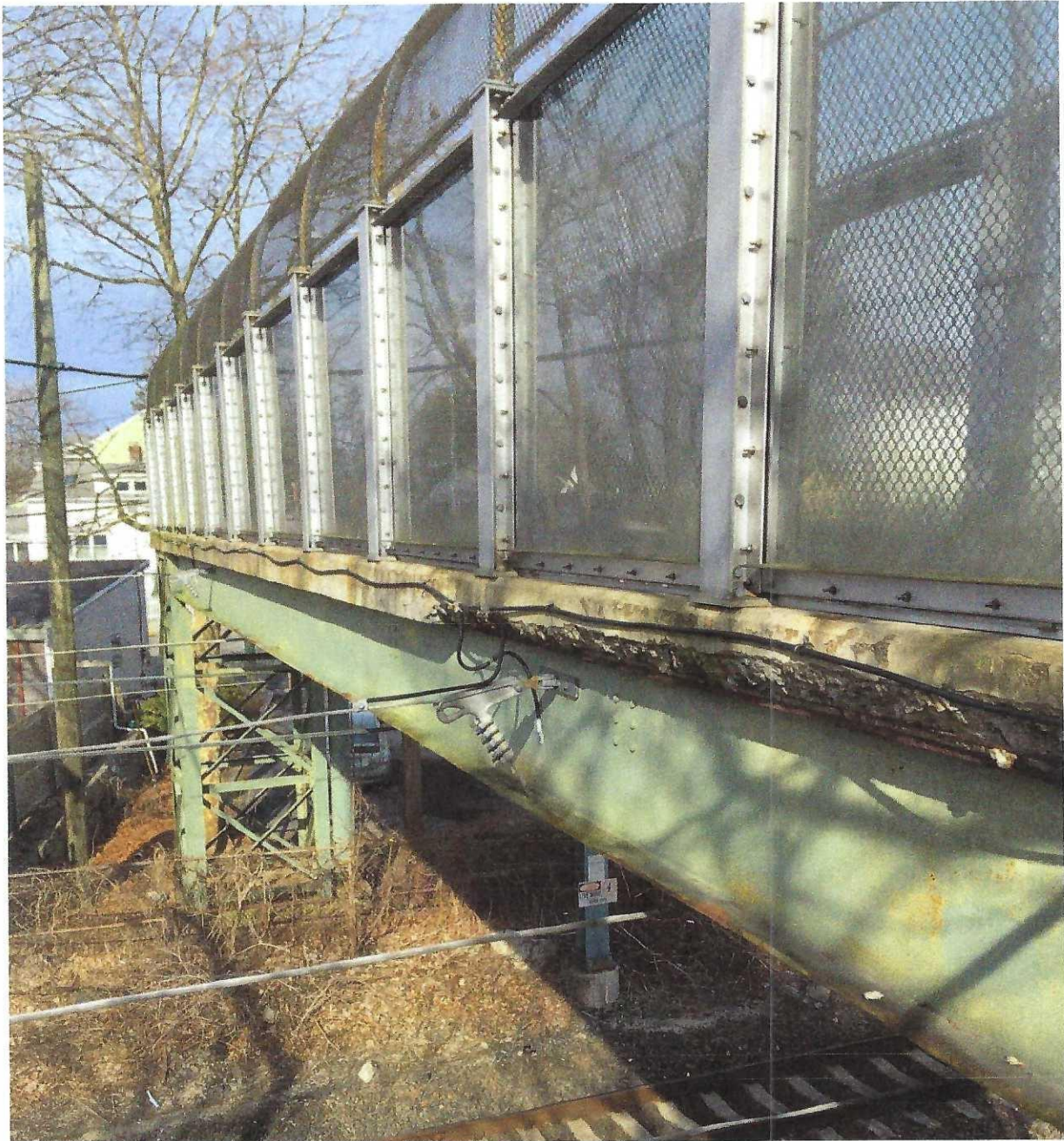
Figure 3 - Northwest side of bridge, looking northeast - Spalled curb
